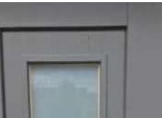
Crack formation, part 2
