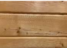
Crack formation, part 1
